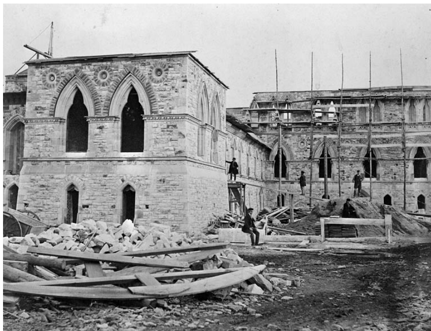
Construction of Parliament Buildings, Centre Block, rear view. Samuel McLaughlin/Library and Archives Canada/C-018016
