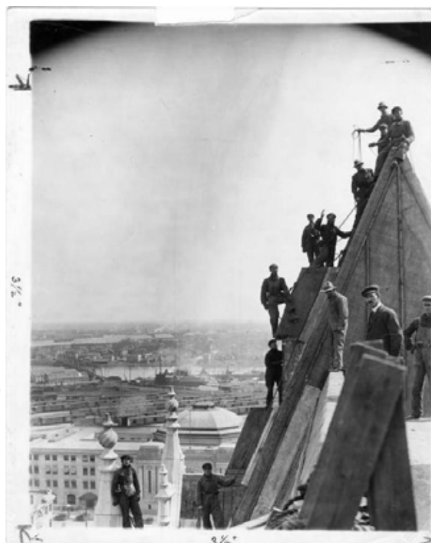
Archives of Manitoba. Lewis B. Foote fonds, 1535. Copper sheathing the roof of the Fort Garry Hotel, 1912-13.
