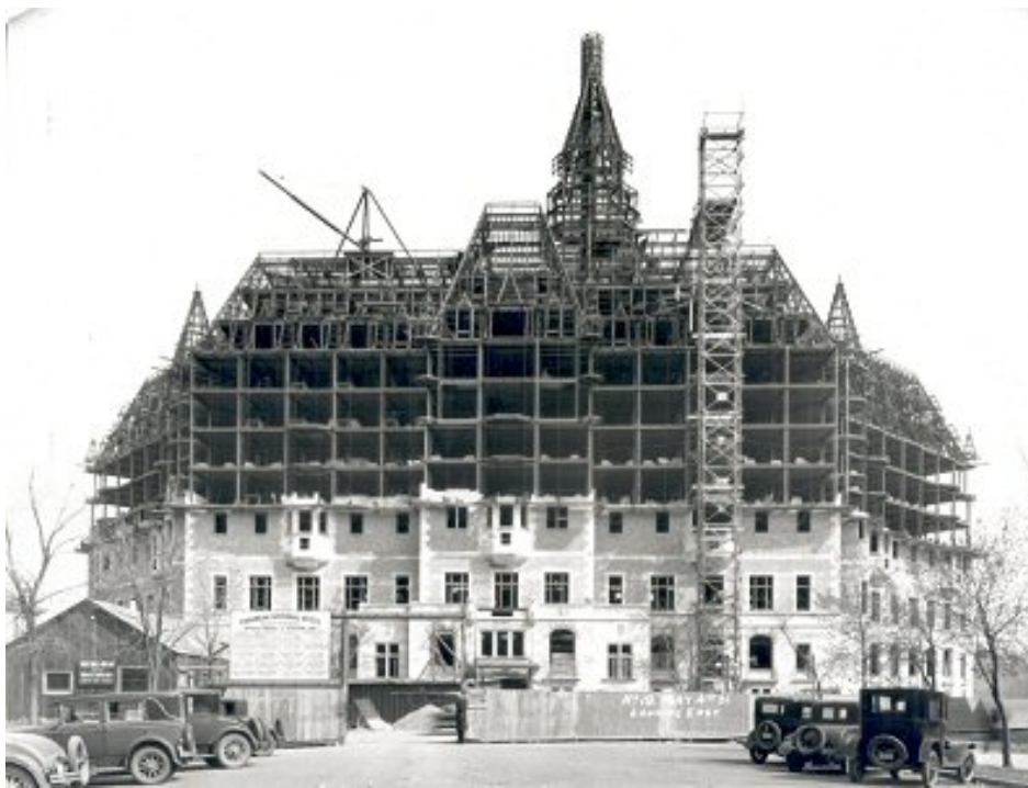
Bessborough Hotel under construction, 1931. Photograph by Len Hillyard. Saskatoon Public Library Local History Room, Hillyard Photographs Collection, A-1351.
